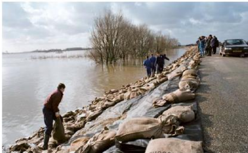
Photo: Emergency repairs with sandbags at Ochten during the high water levels in 1995. Source: Rijkswaterstaat
